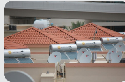
30 VILLA - AL BARSHA (18,000 LITRE HOT WATER STORAGE CAPACITY)
