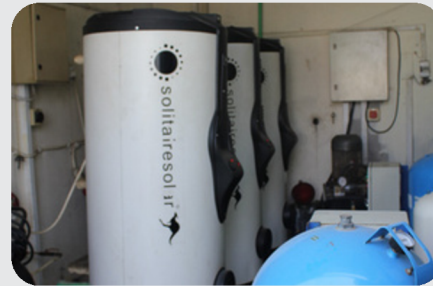
FUJAIRA ABATOIR (6,000 LITRE HOT WATER STORAGE CAPACITY)
