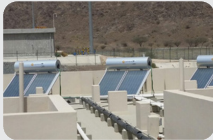
DEWA FACILITY CENTRE - HATTA (1,200 LITRE HOT WATER STORAGE CAPACITY)
